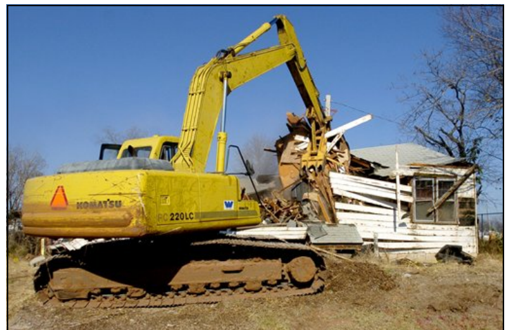
(A crawler excavator tears through the walls of the last house acquired by Oklahoma State University on Tuesday, Nov. 20, 1007, in Stillwater, OK. (Stillwater NewsPress, Mika Matzen)
