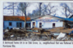
A destroyed home in a New Orleans neighborhood hit by Hurricane Rita.
