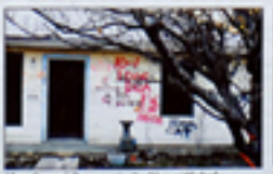
A view of a destroyed home in a New Orleans neighborhood hit by Hurricane Rita.
